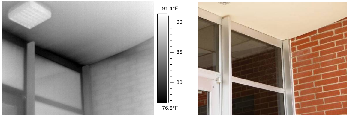
Figure 4 Thermogram and Photograph Pair of Main Lobby Overhang
