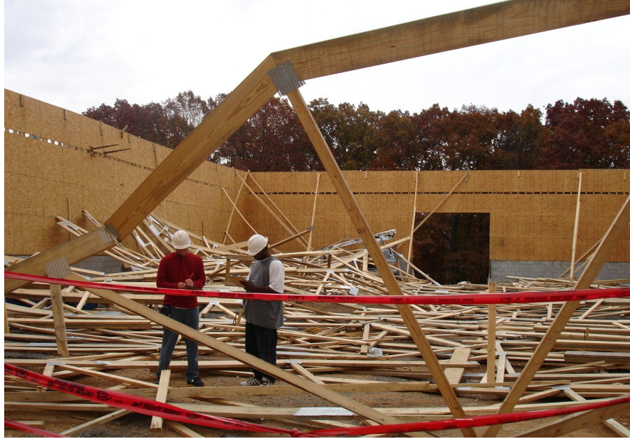
Figure 4: Students taking notes of collapsed trusses
