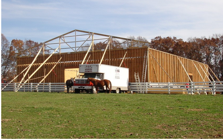
Figure 1: The exterior of the collapsed barn looking north
