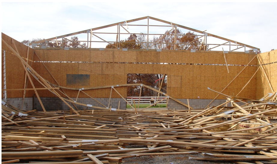
Figure 2: The collapsed trusses looking south
