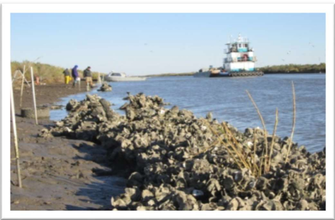
Figure 2. Emplaced biofriendly devices after becoming biologically dominated. These appear and have become part of the environment, and provide sustainable, growing coastal protection.
