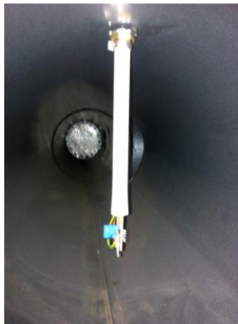
Figure 4. The sensors are fixated at the end of a segment of PEX tubing and the tubing is mounted to the duct wall.
